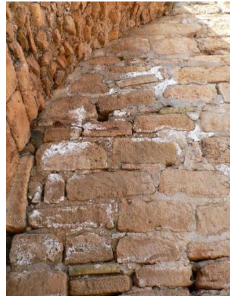
Fig. 4: Damage Salt develops as encrustation covering the stone in interface with cement mortar
