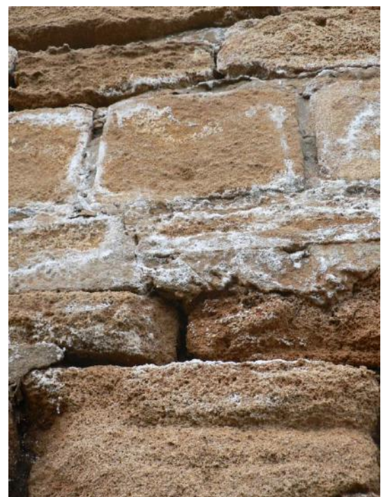
Fig. 5: Details of the saline efflorescences and encrusting on the calcarenite of Salé, at the interface stone-mortar
