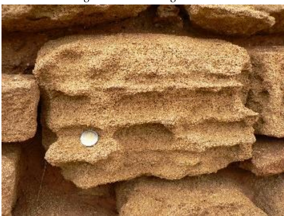
Fig. 7: formation, on the stone surface, of deep interconnected cavities
