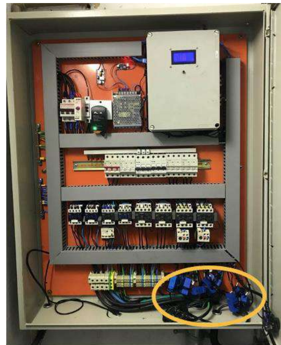
Fig. 2: Electrical panel and current sensors
