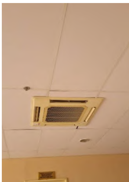
Fig.7 - Split Cassette air conditioning type used in the Lourenço José Ribeiro Forum
