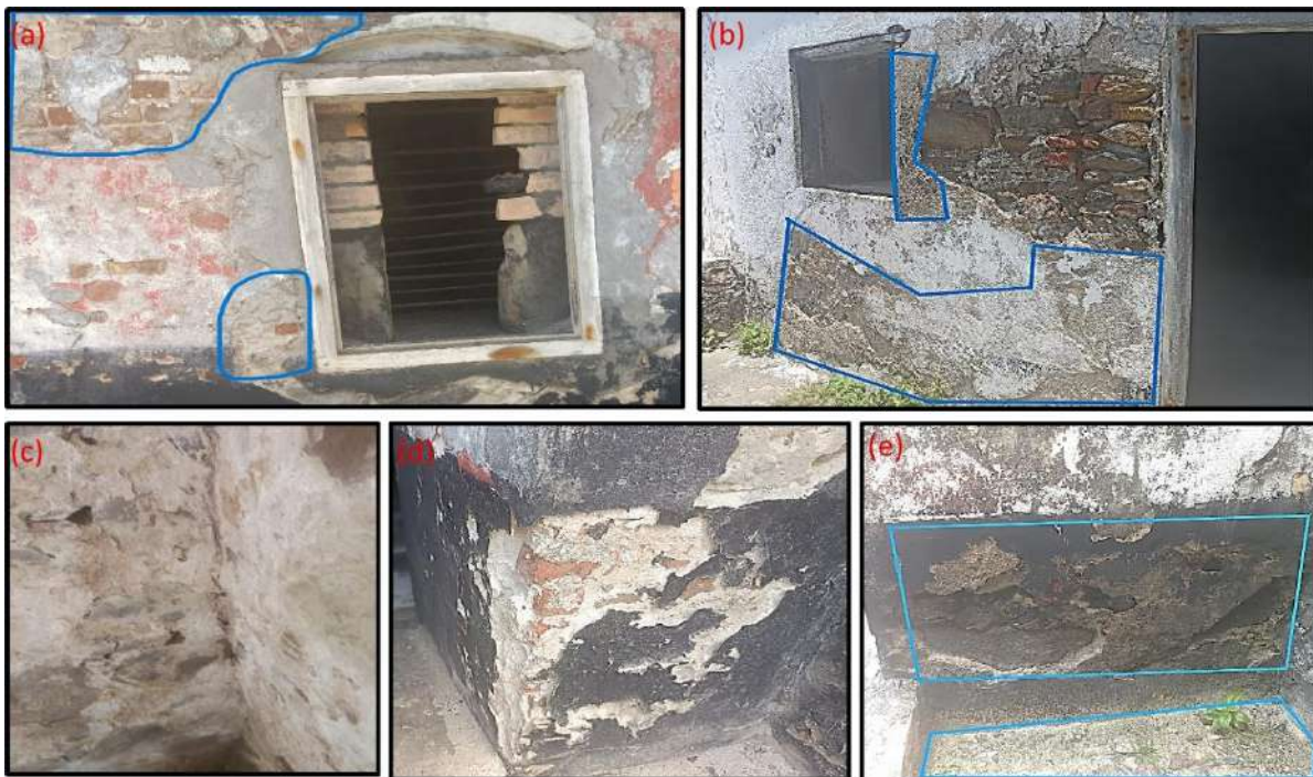
Fig.9a–e: Salt efflorescence, plaster failure and brick disintegration. Source: Site investigation by author; 2025.
