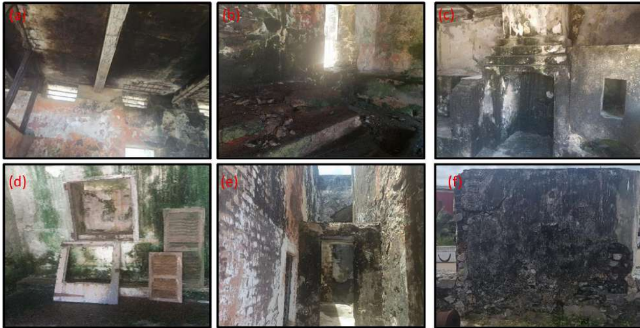
Fig.10a-f: biological colonization. Source: Site investigation by author, 2025.
