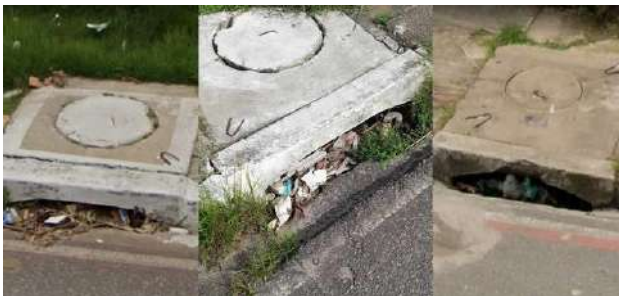
Fig. 10 - Accumulation of solid waste in storm drains.
