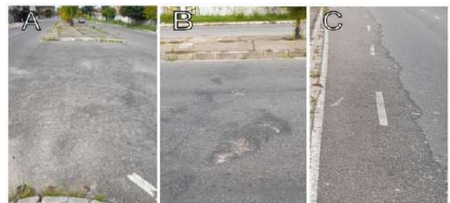
Fig.7 - (A) Wear; (B) Exudation; (C) Surface patch.
