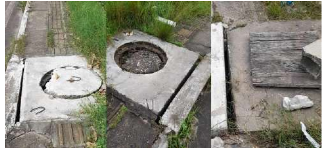
Fig. 11 – Wolf mouths with broken or missing lid
