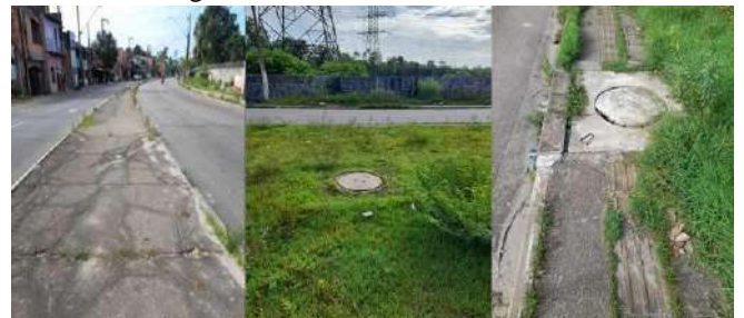
Fig. 13 - Degradation and presence of vegetation on the pavement.
