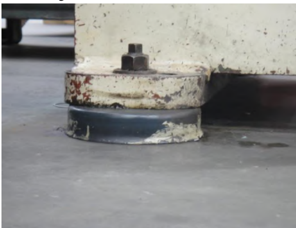
Fig.8: Vibration damper with low efficiency.
