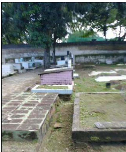
Fig.4: Tomb with masonry perimeter presenting malfunctions. Source: The Authors (2022).
