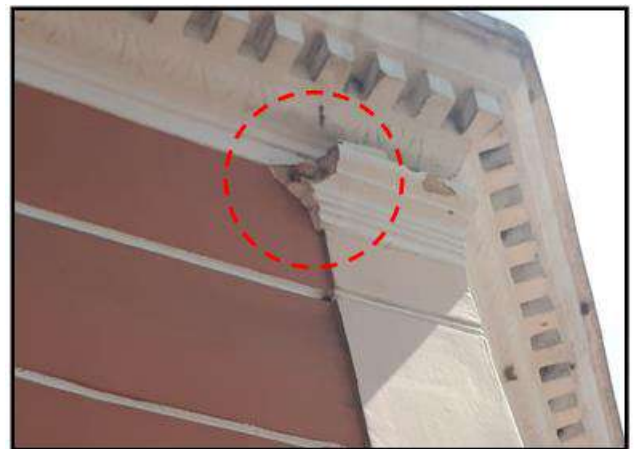
Fig. 7: Areas with loss of concrete
