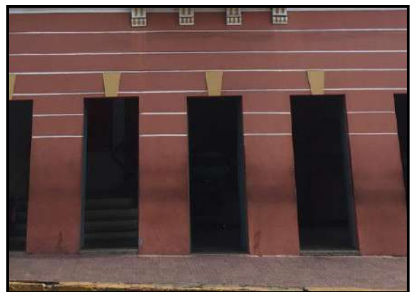
Fig. 3: Surface stains on the facades of the building
