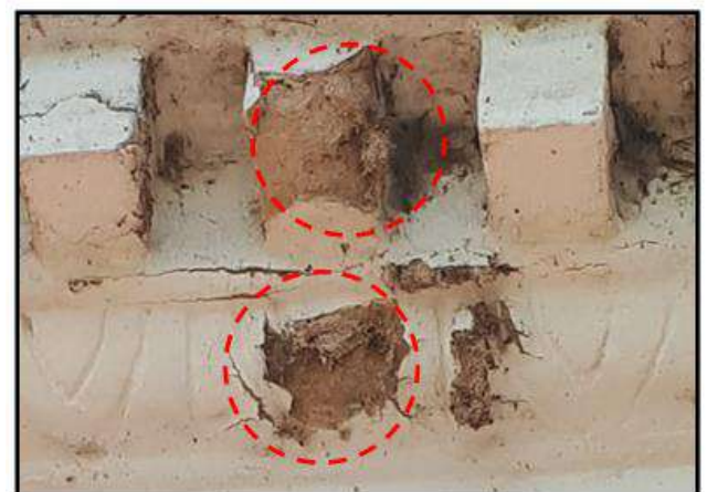
Fig. 8: Areas with loss of concrete
