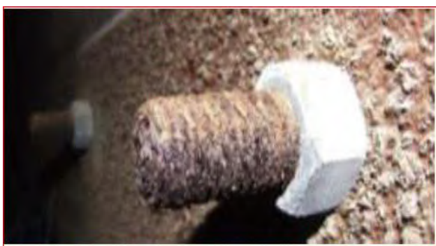
Fig 3 Galvanic corrosion (Mgonja, 2018)
