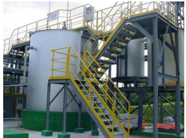
Fig. 7: Effluent treatment plant
