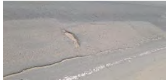
Fig. 24: Pot hole between poorly executed patches (Copyright Images)
