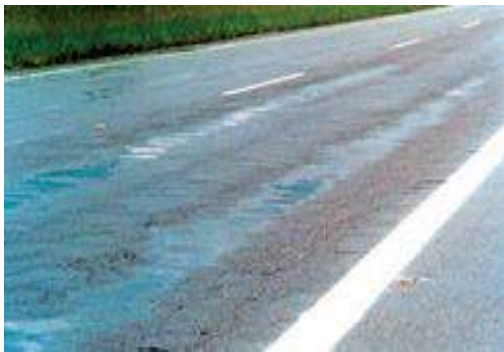
Fig. 7: Sinking by consolidation in wheel track (Inova Civil, 2019)
