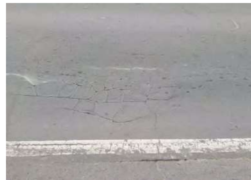
Fig. 19: Alligator cracks (Copyright Images)
