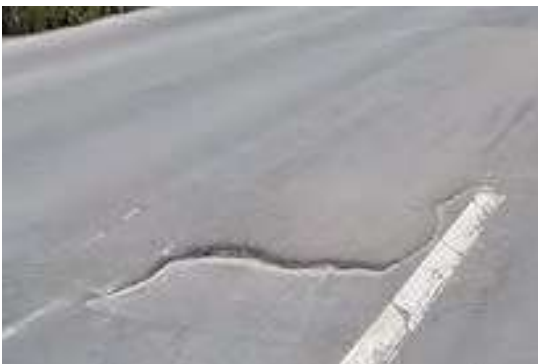
Fig. 23: Patch poorly executed (Copyright Images)
