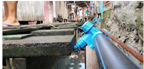
Fig. 3: Aerial water supply network on stilts
