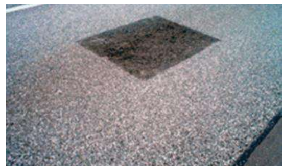
Fig. 16: Patch well executed (Inova Civil,2019)
