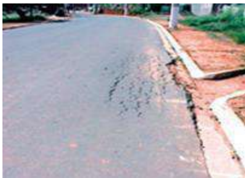
Fig. 8: Localized sinking by consolidation (Inova Civil,2019)
