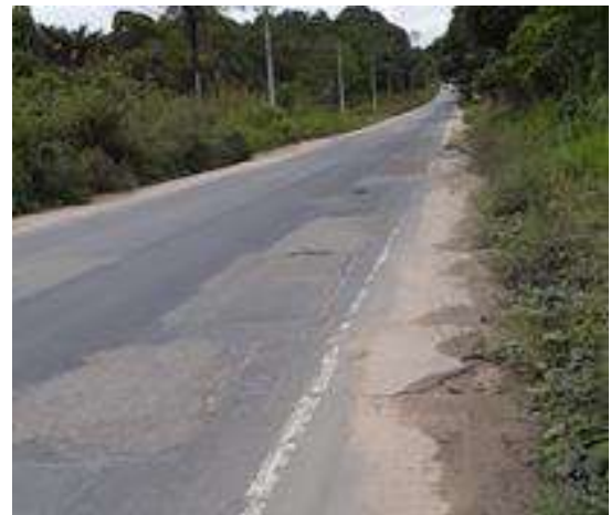
Fig. 25: Patch extension poorly executed (Copyright Images)
