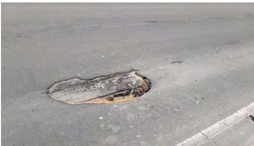
Fig. 22: Pot hole with old patch, reaching the base (Copyright Images)
