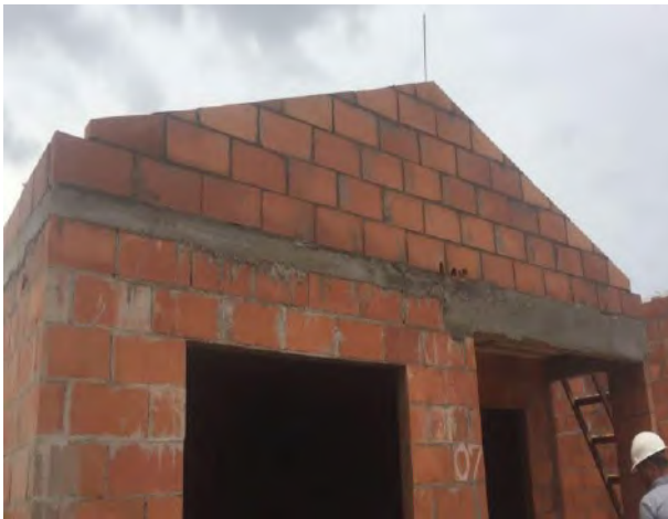
Fig. 6: Details of the construction system in structural masonry, Vila Smart Campo Belo, Iranduba, Amazonas.
