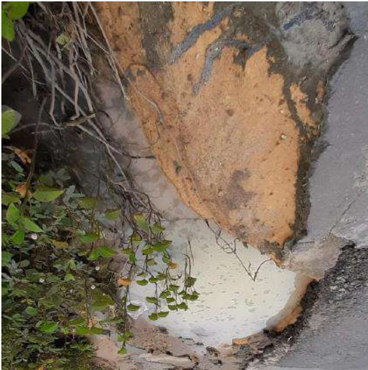
Fig. 21: Pot hole reaching the base, on the sideway (Copyright Images)
