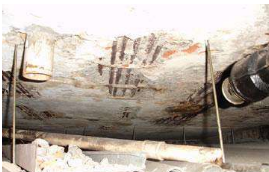
Fig.4: Pathologies arising from lack of waterproofing.
