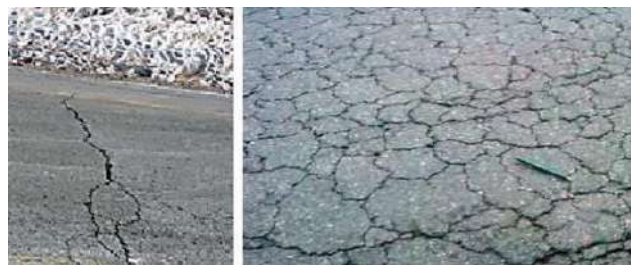
Fig 11 Alligator skin crack, Bernucci et al.(2012)
