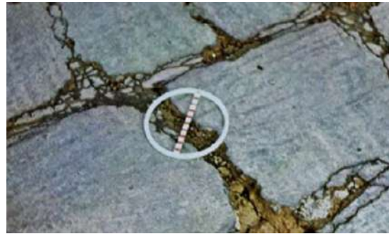
Fig. 5: Block crack (CNT, 2019)
