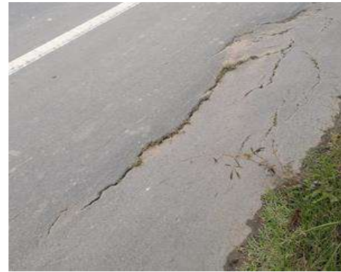
Fig. 18: Longitudinal cracks (Copyright Images)
