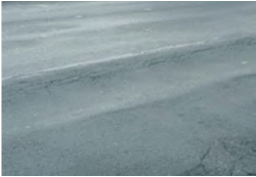
Fig. 6: Plastic sinking on wheel track (Inova Civil,2019)
