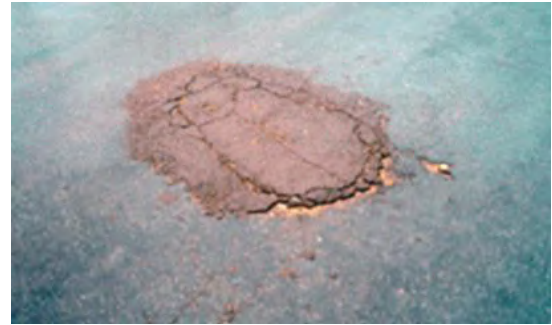
Fig. 15: Poorly executed patch (Inova Civil,2019)
