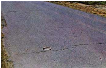
Fig. 2: Transverse crack (CNT, 2019)
