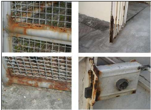
Fig. 9 - Intense corrosion of the gates and the lock
