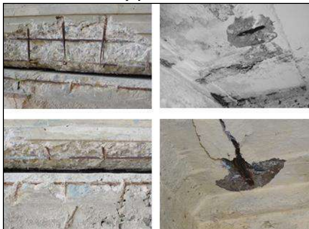
Fig. 5 – Aspects of corrosion in the reinforced concrete viaduct
