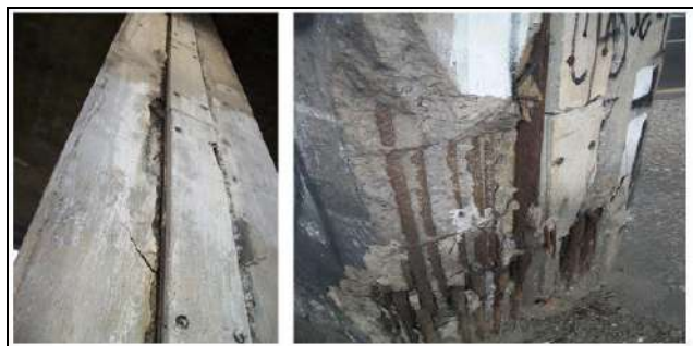
Fig.6 – Aspects of corrosion in the reinforced concrete viaduct
