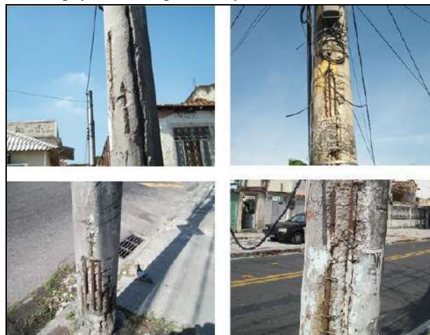
Fig. 7 - Aspects of intense corrosion of public lighting poles
