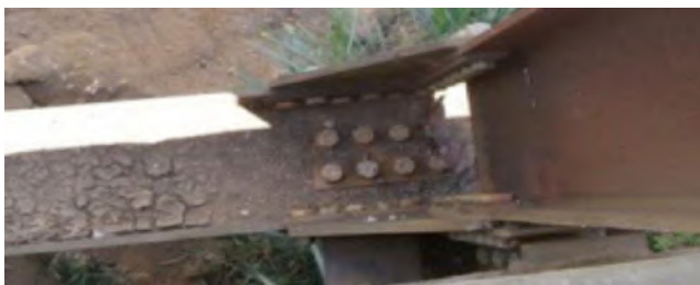
Fig 8.- Accumulation of sediments in the lower string of the truss (Bridge over the Pirris River - National Route 226)
