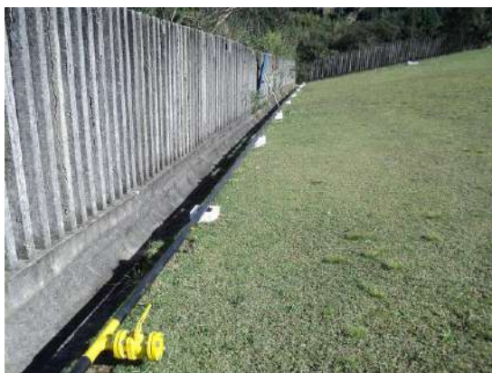
Fig. 5: The main pipeline
