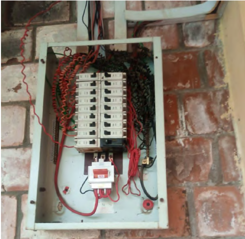
Plate 6: Image Showing Existing Exposed Electrical Control Box Imposing Risk to the Occupant of Silver Hostel Facility, Bellstech
