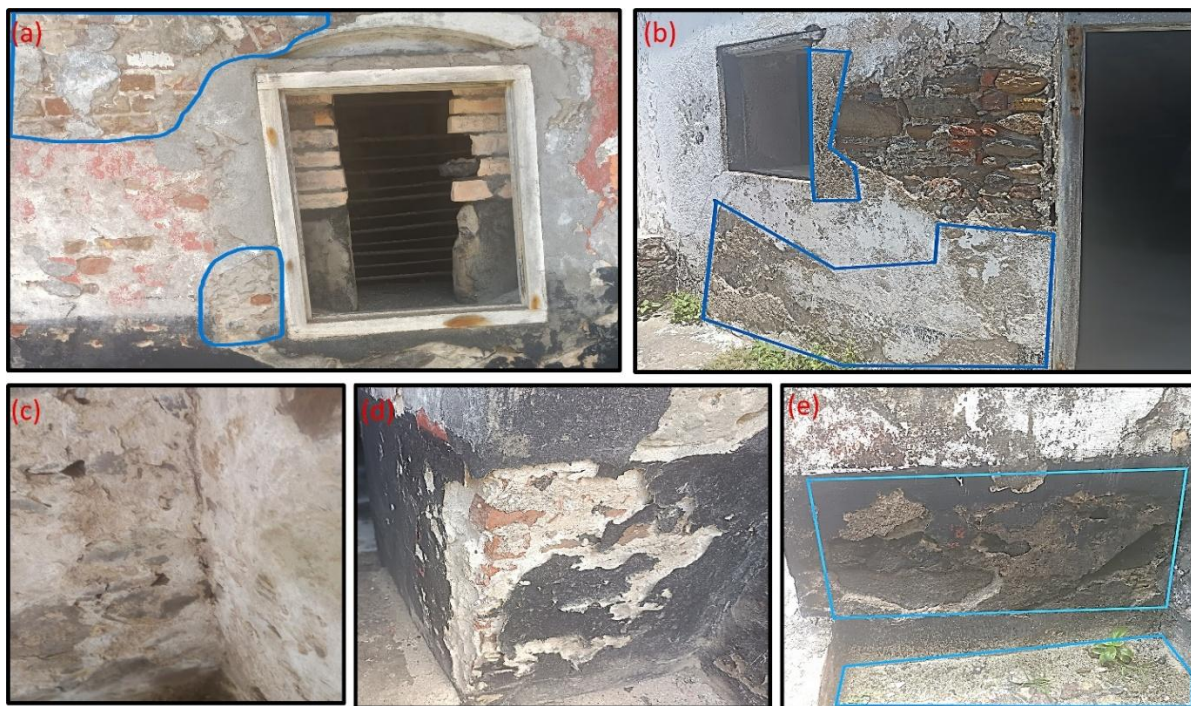
Fig.9a–e: Salt efflorescence, plaster failure and brick disintegration. Source: Site investigation by author, 2025.
