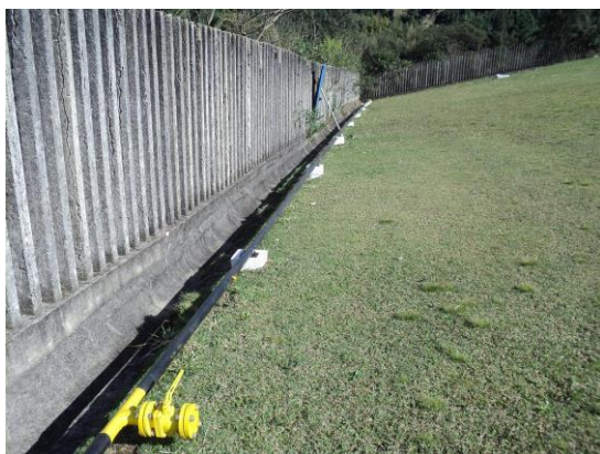
Fig. 5: The main pipeline
