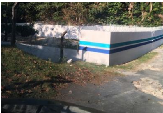
Fig. 6: Sewage treatment station
