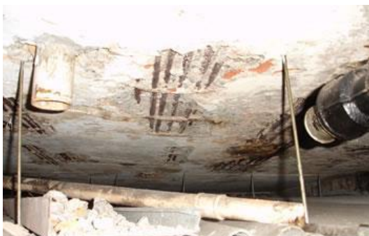
Fig.4: Pathologies arising from lack of waterproofing.
