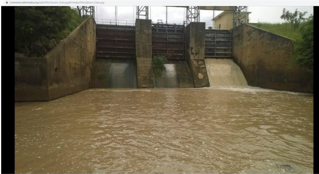
Fig.2: Image of the Ojirami dam source of water distribution to the network
