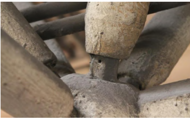
Fig. 3-8: Bolt sleeve pin is missing
