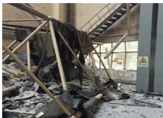
Fig. 3-6: The collapse of the scene
