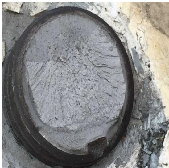
Fig. 3-13: M33 high strength bolts fracture
