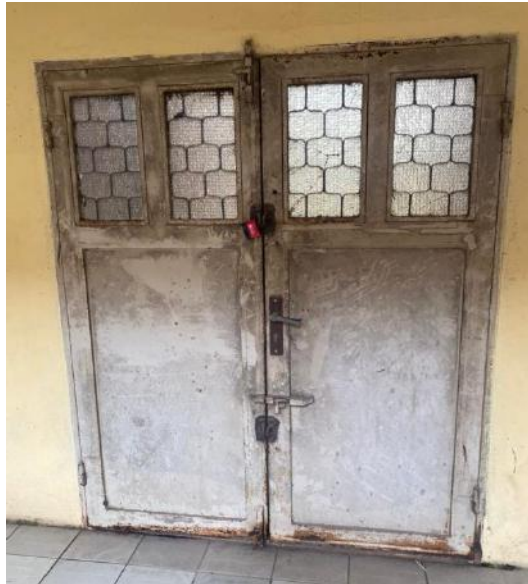
Plate 3: Image showing the fire escape door, brick wall, and escape staircase in the building.
