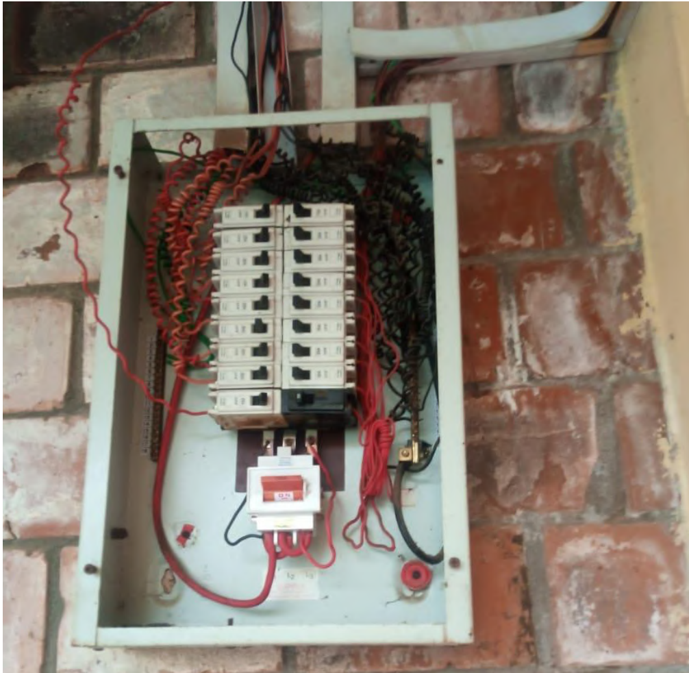
Plate 6: Image Showing Existing Exposed Electrical Control Box Imposing Risk to the Occupant of Silver Hostel Facility, Bellstech
